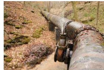
Figure 1: A Trivial Water leakage Location
